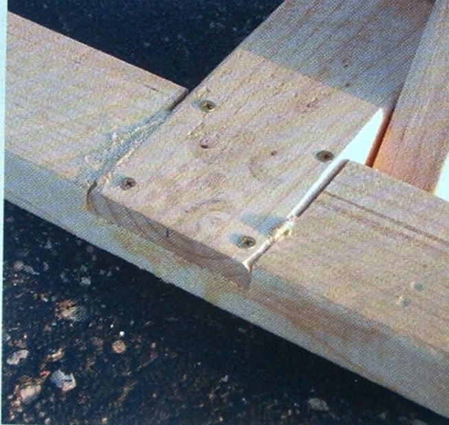
The joints of the base are laps, cut by table saw and secured with glue and wood screws.
