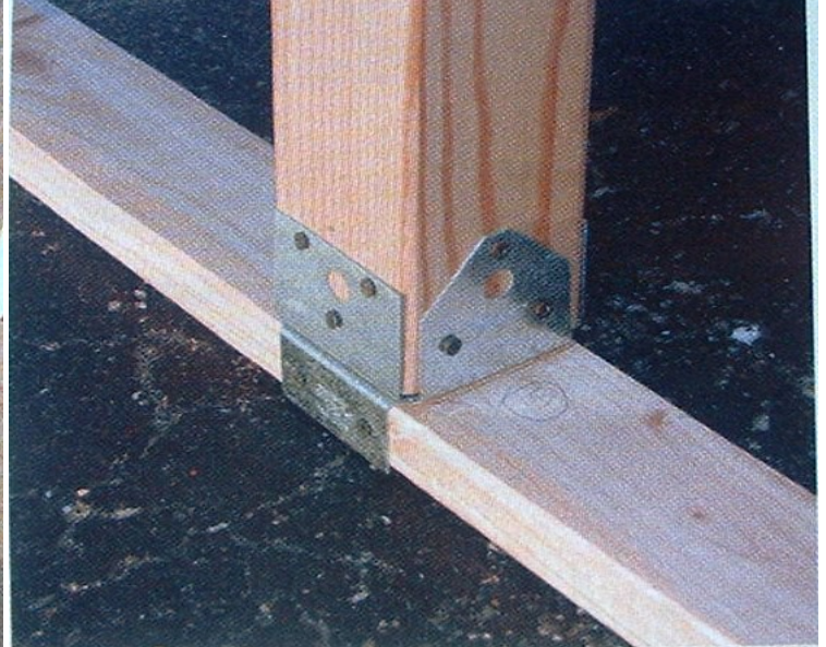
The vertical support post is mounted and stabilized with wooden braces, braided wire cables, and aluminum deck-post brackets.
