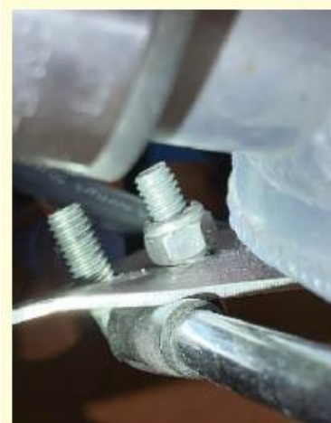
Missing nut on U-bolt
